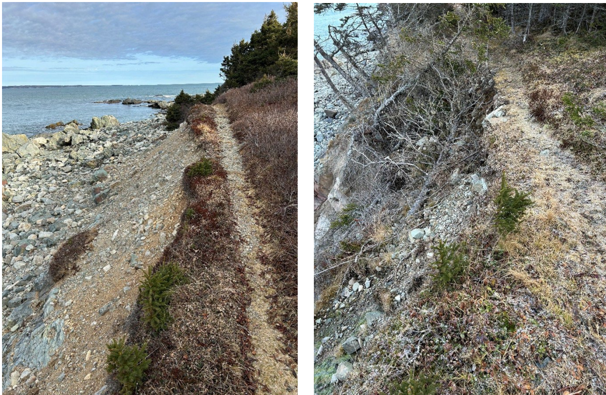
Figure 3: Gull Cove Trail showing coastal trail sections being undercut by coastal erosion (2023)
