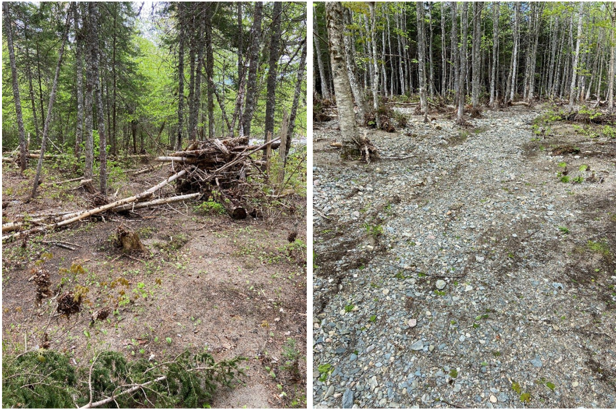
Figure 6: North River Falls Trail showing surface erosion and debris piles in a floodplain zone.
